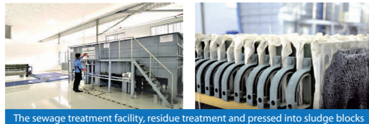
The sewage treatment facility, residue treatment and pressed into sludge blocks
